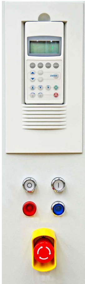
Figure 8-1 ARU control panel
